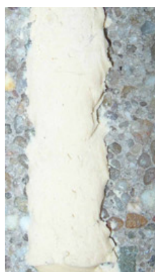
Cohesive failure in adhesive
